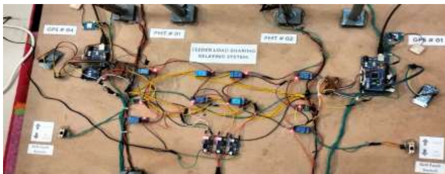
Figure 8: Monitoring, Protection and Automatic Fault Management Devices Installed on PMT Secondaries of the distribution network
